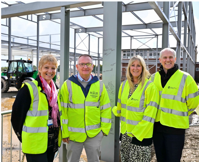
Marking a milestone: Gillian Elliott from the Nuclear Decommissioning Authority, David Savage, Chair of Town Deal Board, Kelly Anderson from South Copeland GDF Community Partnership and Paul Skelton from Nuclear Waste Services
